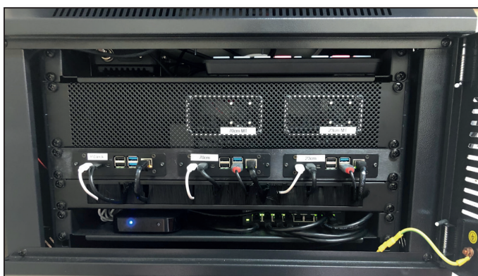
► Figure 1: The GB3JV Transmitter Input Equipment (TiE) Bay
